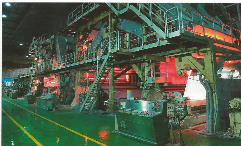
Fig. 2: Compact Engineering's IRE at the 1st and 2nd coater head in the foreground, Impact's emitter on the top coating in the background
